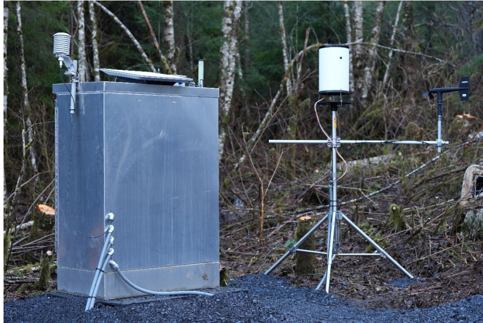
Figure 1 - Avionics Cabinet and Weather Station WEMA2
