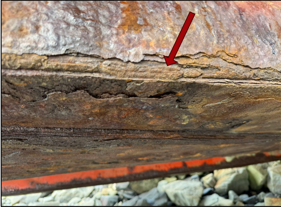
FIGURE 11. Corrosion and loss of weld material along bottom flange edge at web junction.
