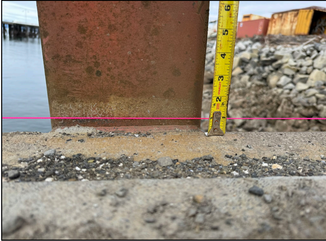
FIGURE 17. Sag at mid-span of the barge ramp (i.e. ramp bent due to overloading).
