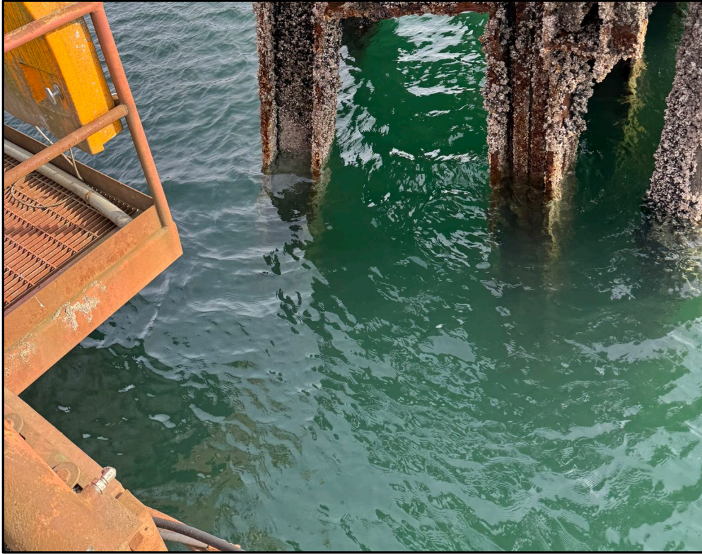
FIGURE 7. Tether cable missing/detached from barge ramp on south side.
