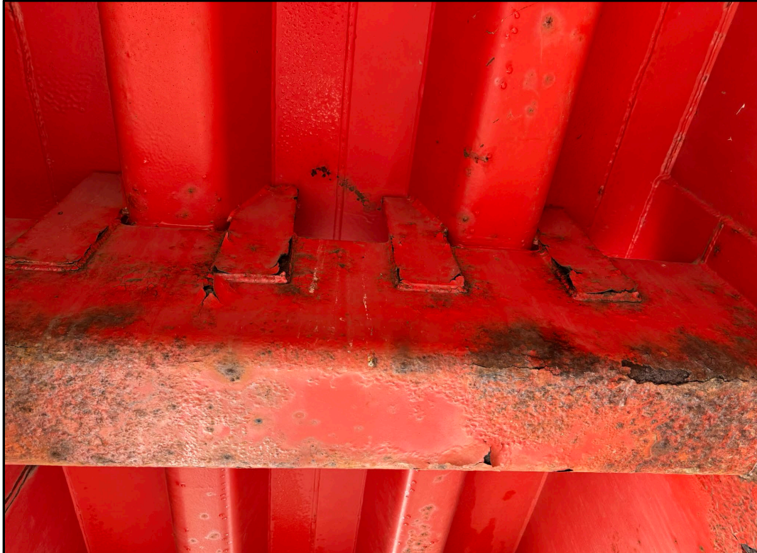
FIGURE 14. Typical coating failure and advanced corrosion of ramp floor beam.
