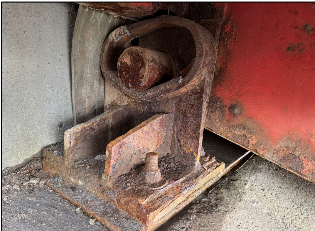
FIGURE 12. Corrosion at abutment bearing assembly; deformed/repared saddle bearing.
