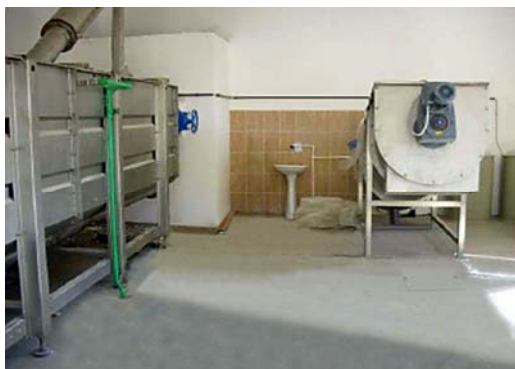
XMD 70 ÖÜÿÔCSÒÁÜÜÒÙÙ with TOP 3 Combined Screen, Grit and FOG removal plant installed inside a purpose-built building
