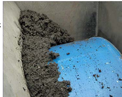
Dewatered dry solids conveyed into the ÖÜÿÔCSÒÁÜÜÒÙÙ discharge section
